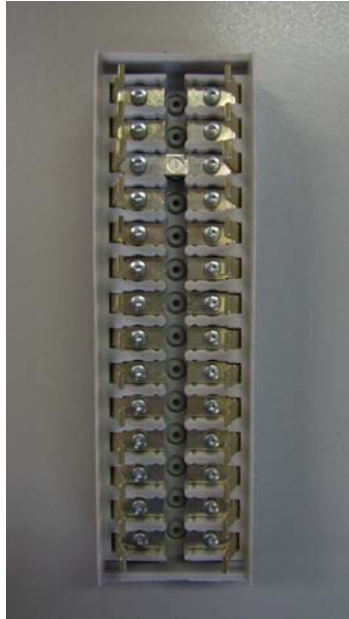
Outer case terminal block showing CT shorting link across terminal 5-6.
